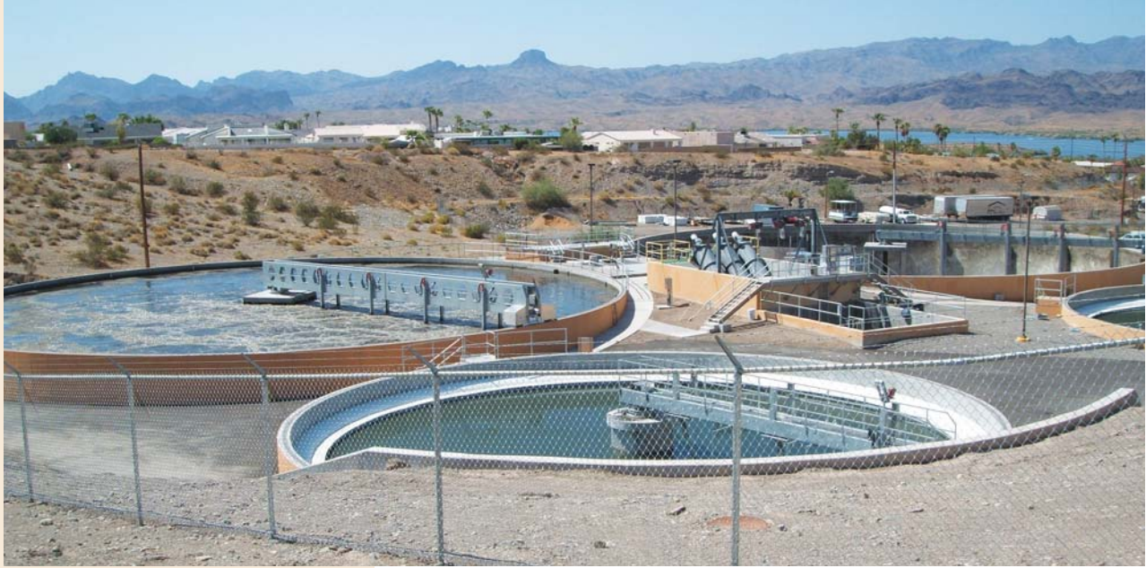
Upgrades and expansions to Lake Havasu City's wastewater treatment and collection systems have made it possible to supply three area golf courses with irrigation water that is safe and affordable.
